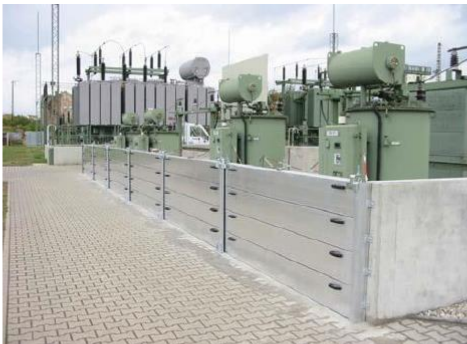
Figure 6.5: removable flood panels (ENA ETR138 Annex 1)
